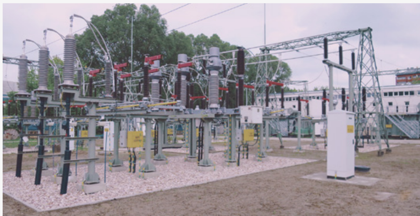
innogy Stoen Operator, RPZ Stodowiec 110 kV
